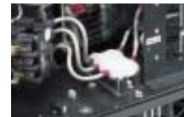
Coated Electrical Connections
