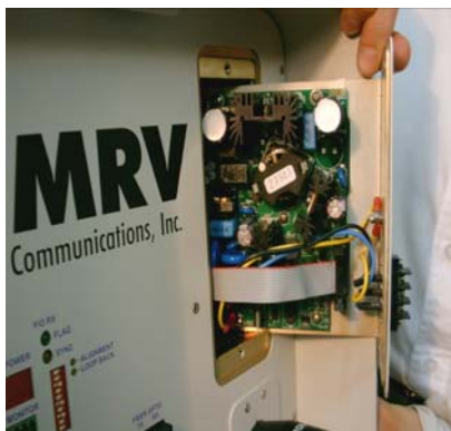
Figure I.2: Pulled out Power Supply
