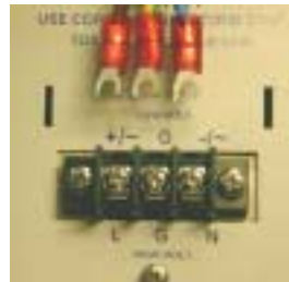
Fig. 6.4: Power cable & Terminal block
