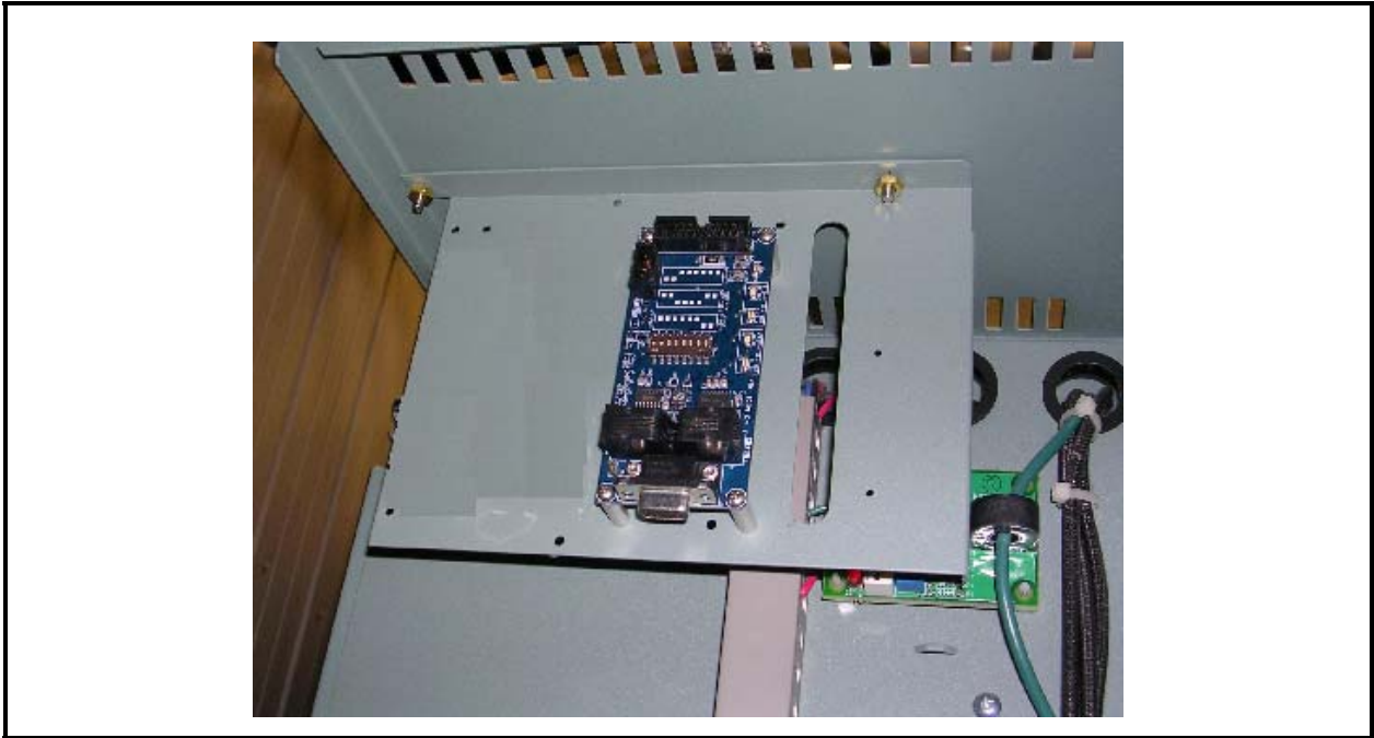
Figure 3. NHD1 LINKS 2 Slave Installation
