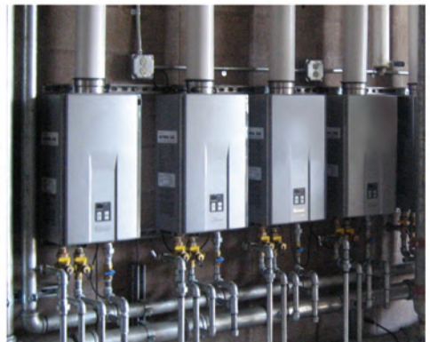
High school expands available space in mechanical room with increased efficiency and less capital expense.
