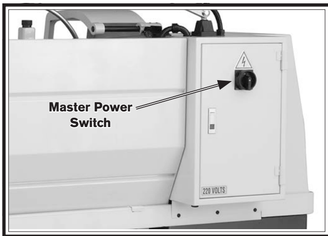
Figure 28. Location of the master power switch.
