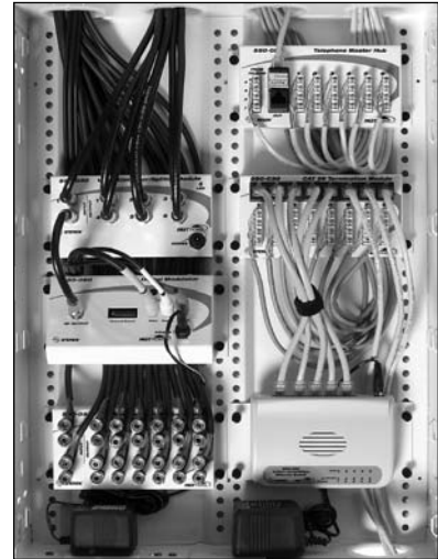
Sample configuration for telephone, audio/video, security and Ethernet.
