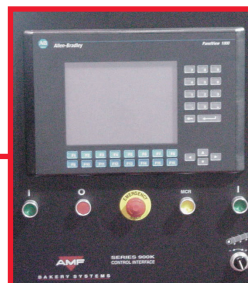
Operator Interface Panel
